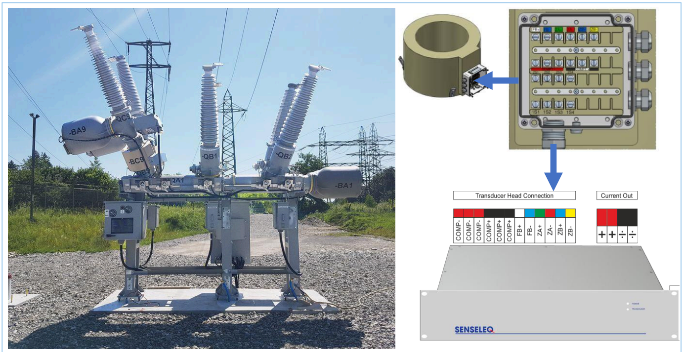
Figure 13: Fluxgate current transformers on GE's HYpact switchgear
