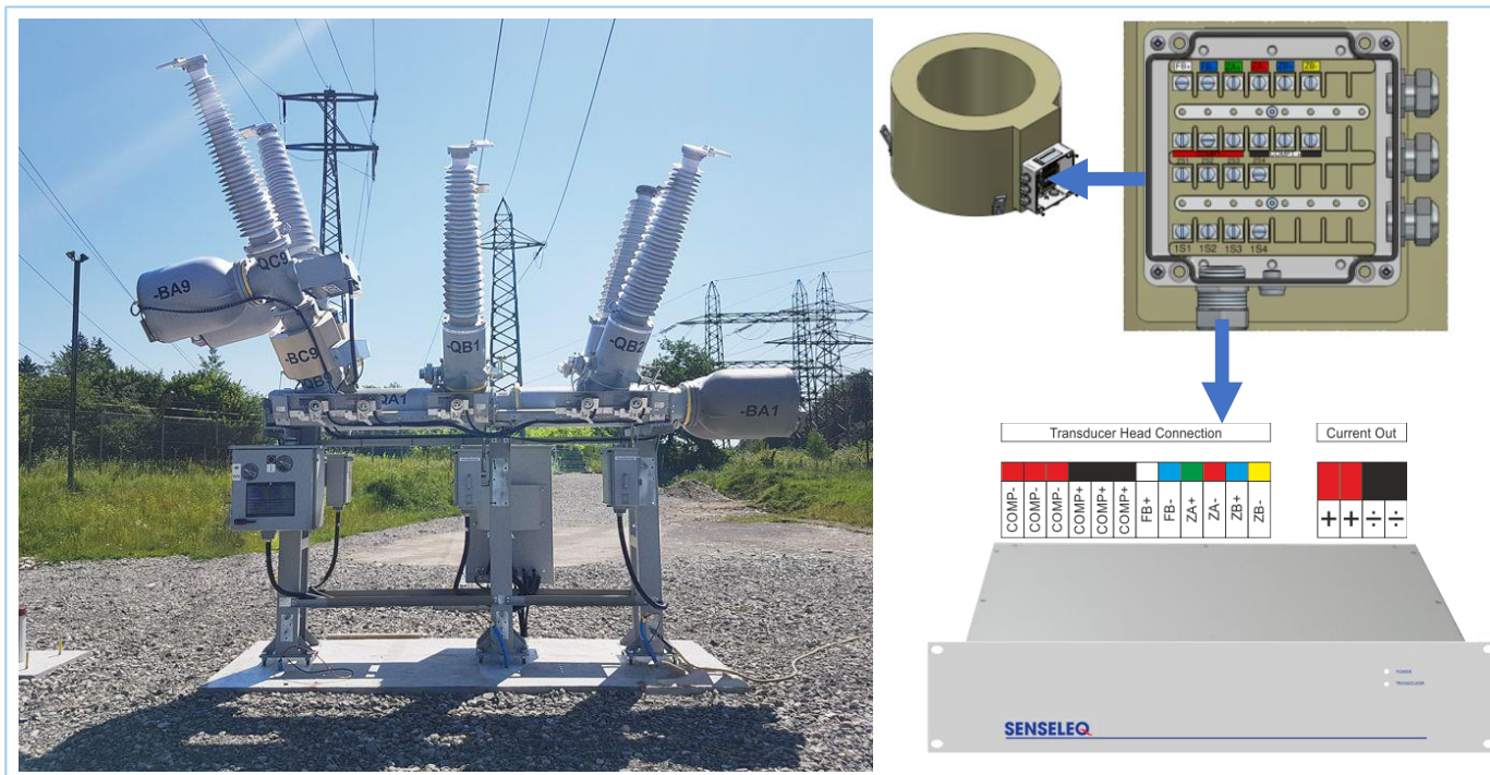
Figure 13: Fluxgate current transformers on GE's HYpact switchgear
